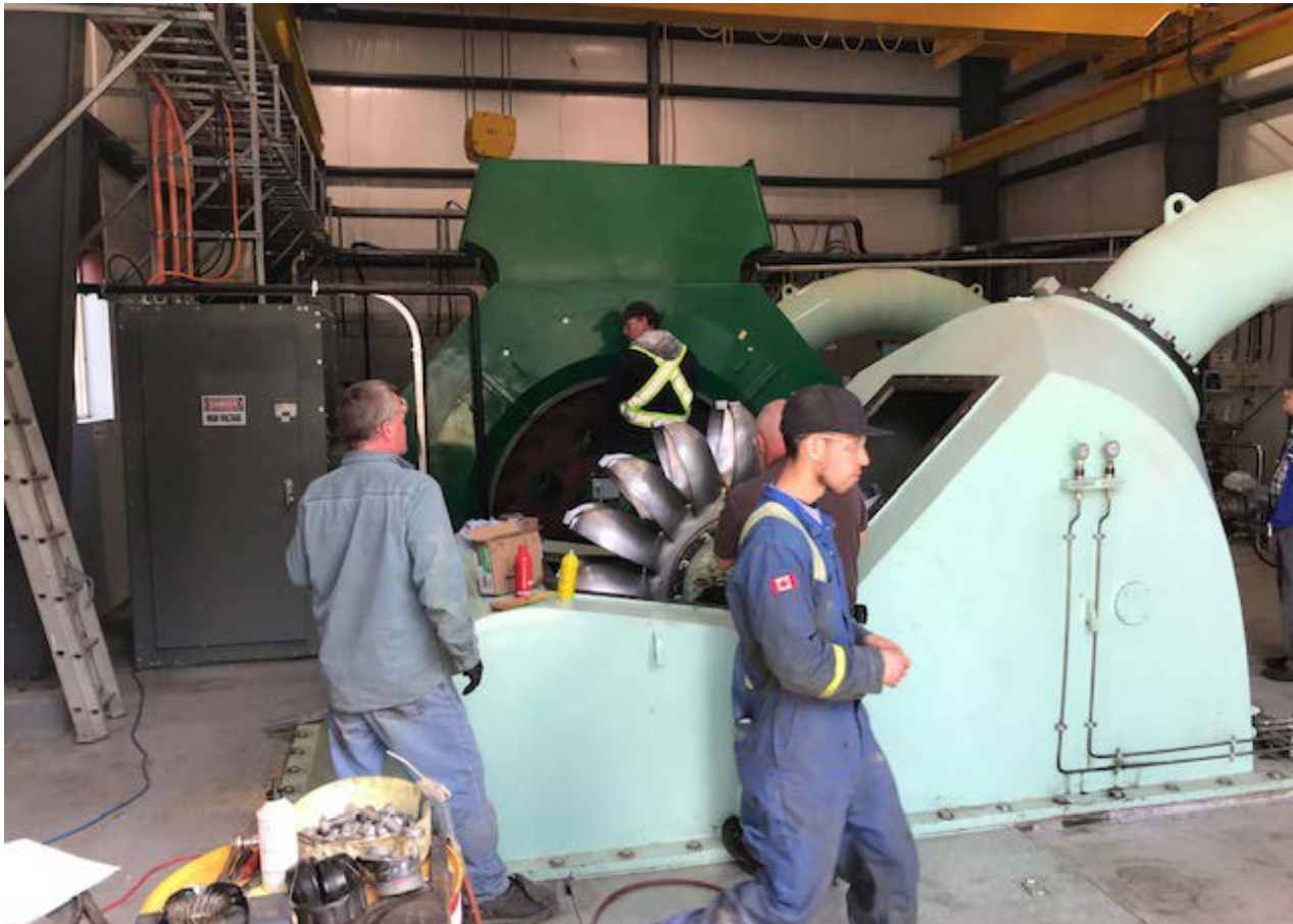
Pelton turbine in existing powerhouse.
